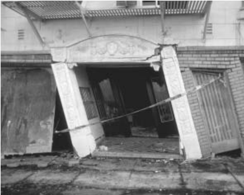
Entrance and garage level of a Beach Street apartment complex in danger of collapse after the 1989 Loma Prieta earthquake, Marina District.
